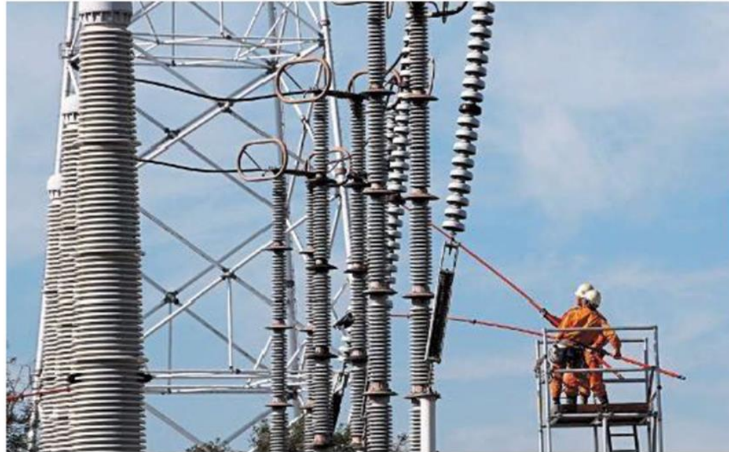
Rising costs: Men working at a transmission tower in Kakogawa. Japan's domestic fuel and power bills have reached a four-decade high. — Reuters
